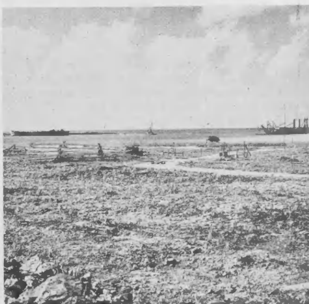
THIS IS the site where the chemical complex at Barcadera will be constructed. At right is the business end of the cutter-suction dredge "Barlow," which is expected to finish the industrial harbor dredging operation in about three months.
